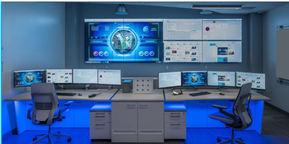
Figure 4. The Architecture of NOC and SOC Operation Room.
